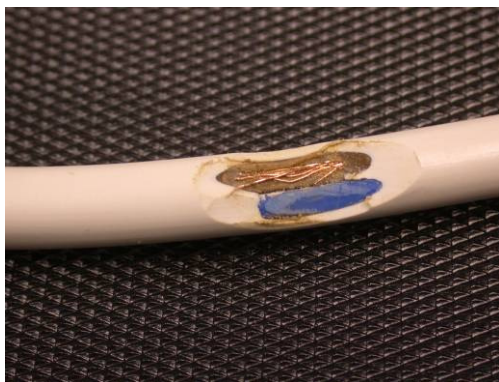
Damage to power cable sheath.
