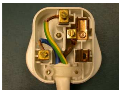
Bare wires visible
