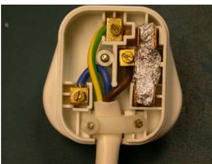
Fuse not being used
