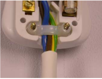
Cable not being gripped
